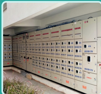
LT METERING PANELS
